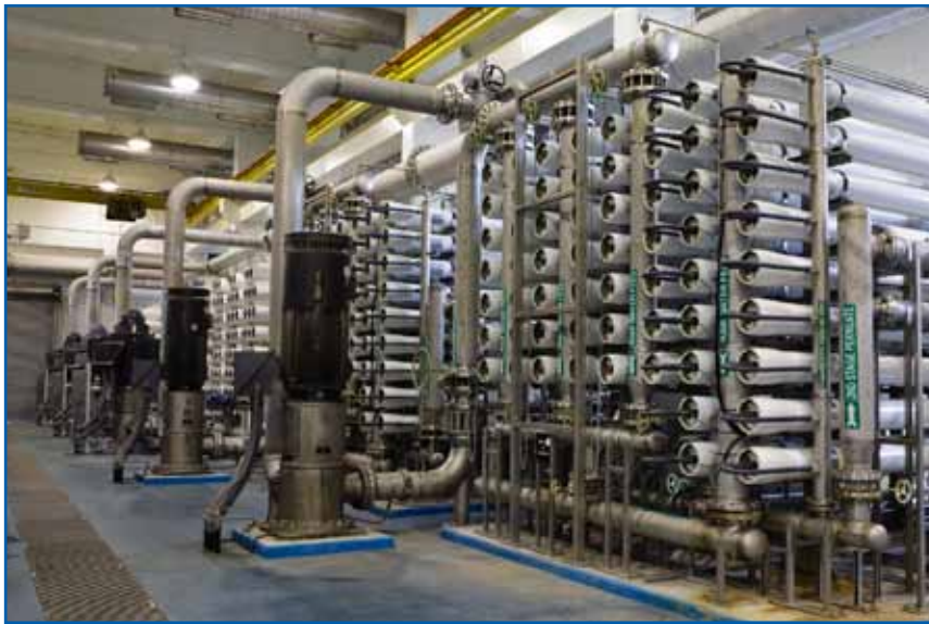
Public utility reverse osmosis water treatment plant includes multiple spiral wound membranes
