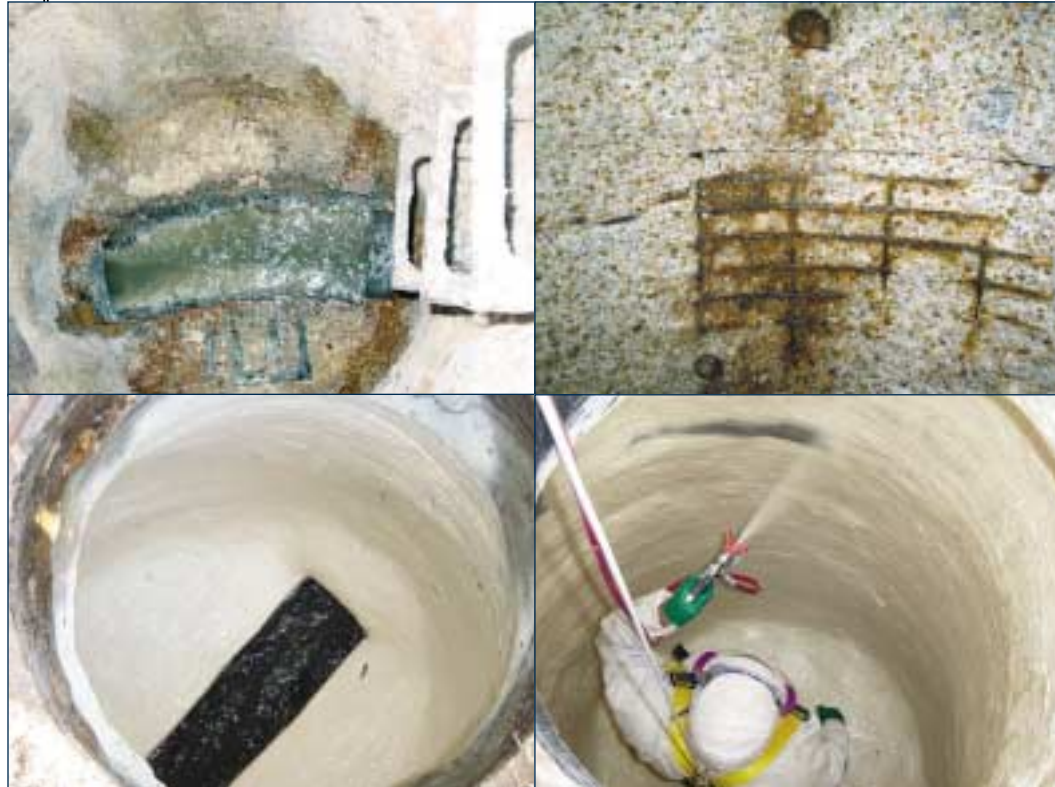
Manholes have proven to be prime candidates for Zebtron applications by PIC. Clockwise, from top left: steps are loose and corrosion is evident in this manhole; blasting reveals steel supporting the concrete walls; Joyce sprays Zebtron; the finished manhole.
